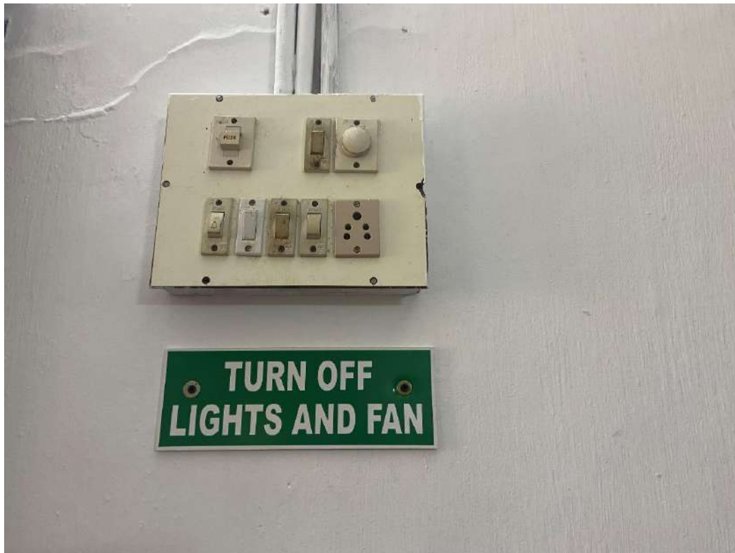
Turn off lights – stickers on switch boards
