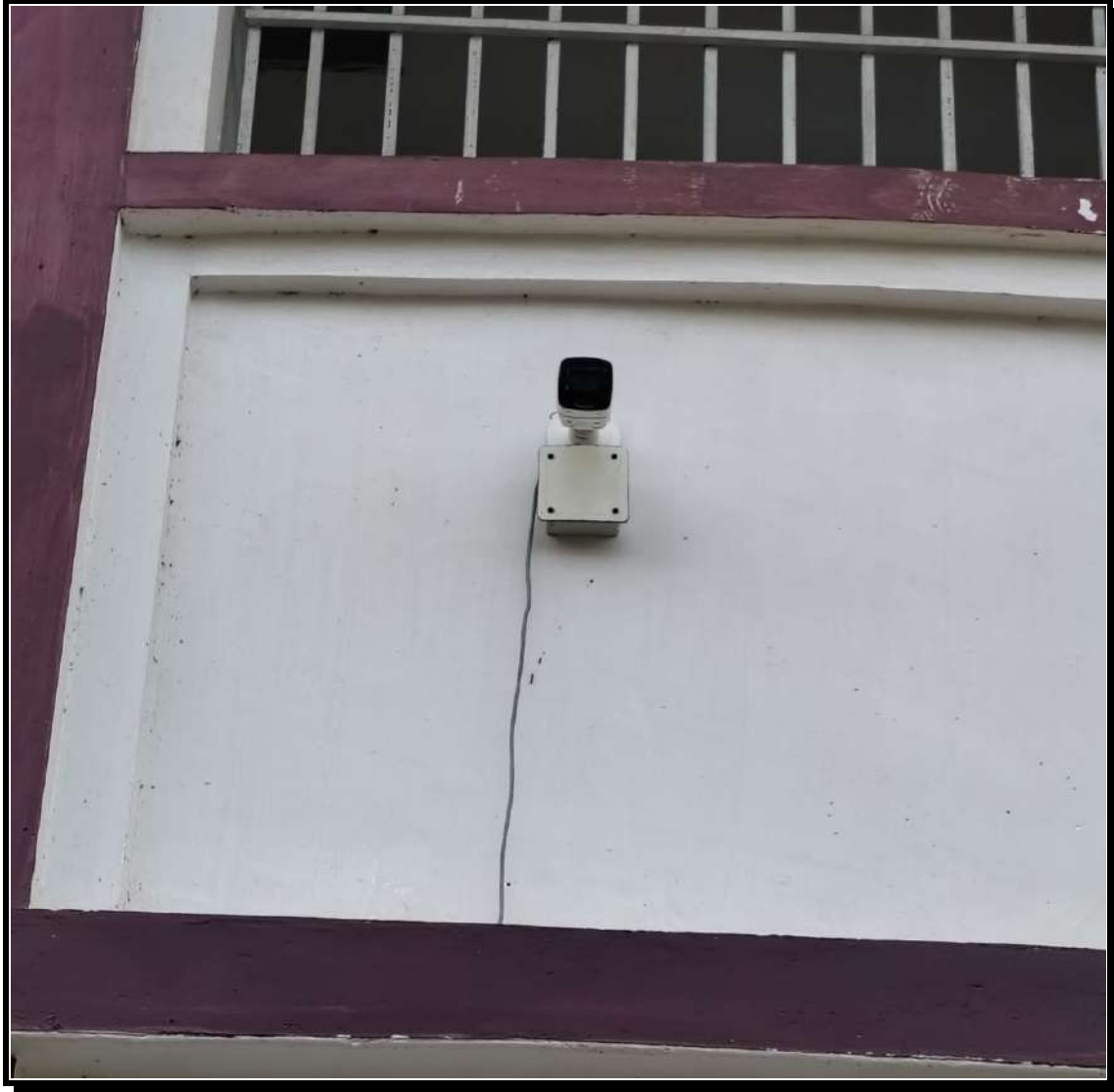
Figure 15: Advanced Night Vision Cameras Ensuring Safety inside Campus and Premises
